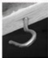
Ceiling "J" hook centered on joist
